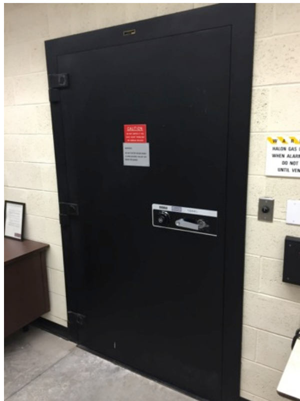
Example: High Security Vault
